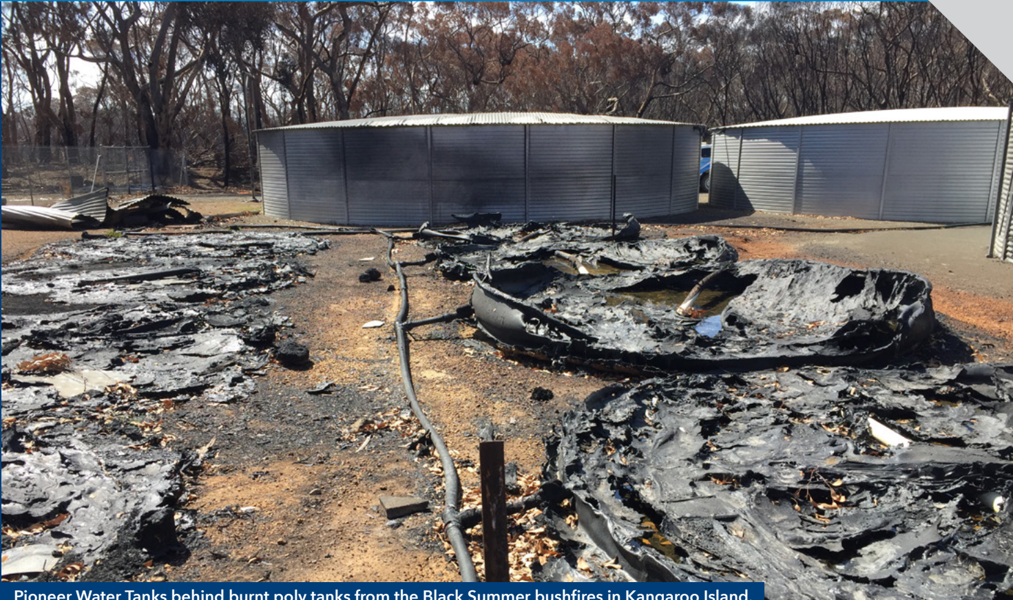
Pioneer Water Tanks behind burnt poly tanks from the Black Summer bushfires in Kangaroo Island.
